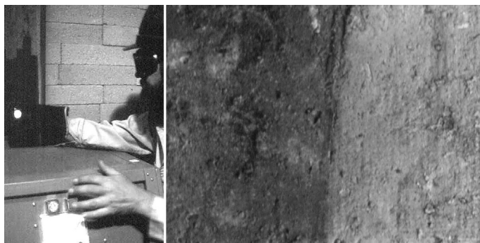
Fig. 2. Xenon flashlamp surface ablation in air of contamination on a steel beam (left). Concrete surface contamination on left and flashlamp divested region on the right side. (right)
